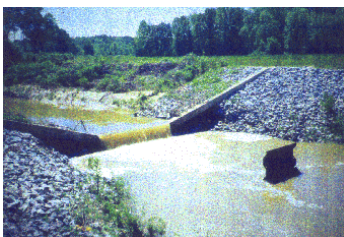
Low drop elevation weir
